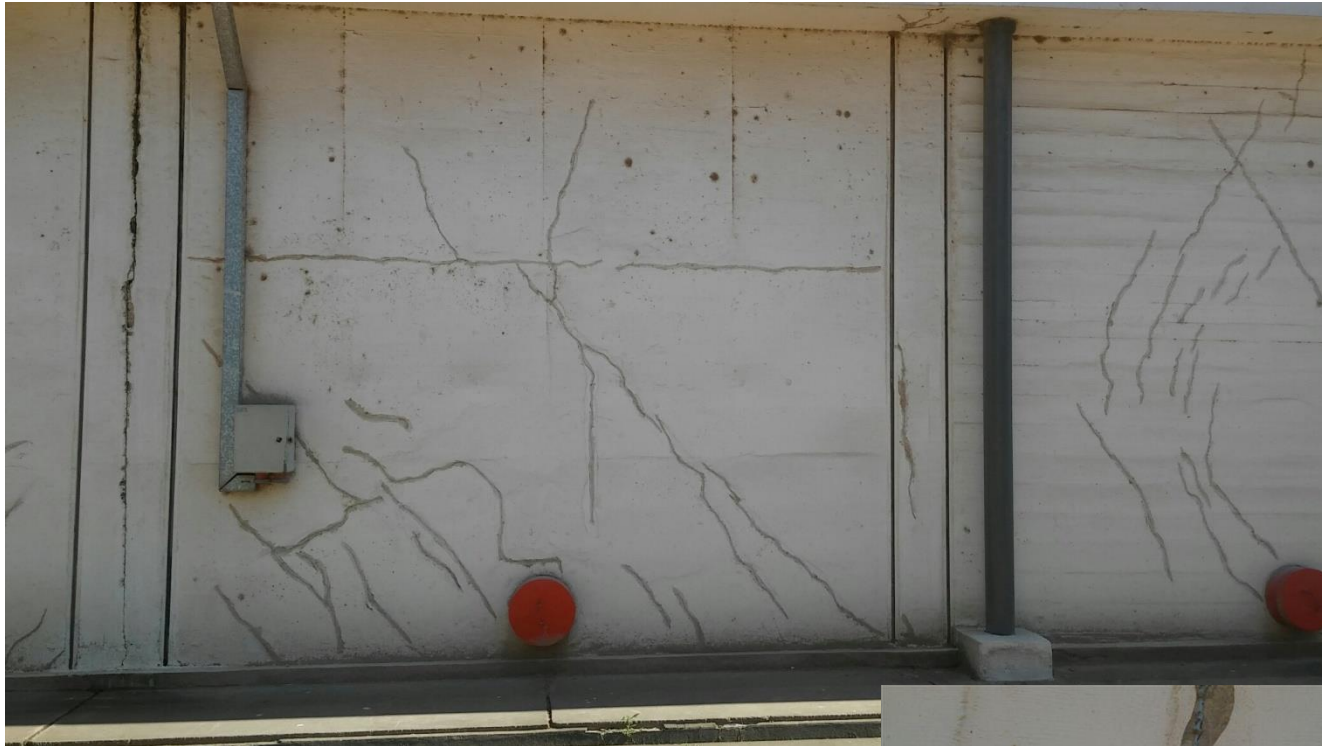
CRACKS IN SILO WAREHOUSE WALL DUE TO OVERLOADING
